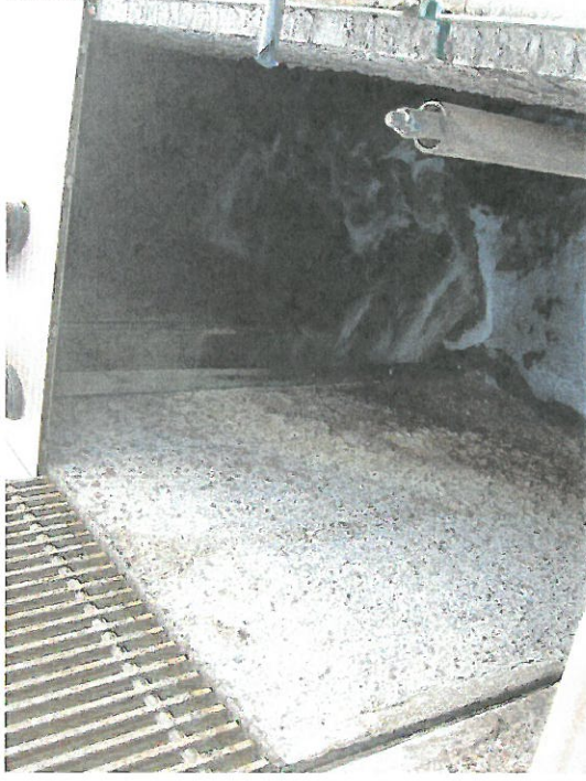
Primary Clarifier Flow
