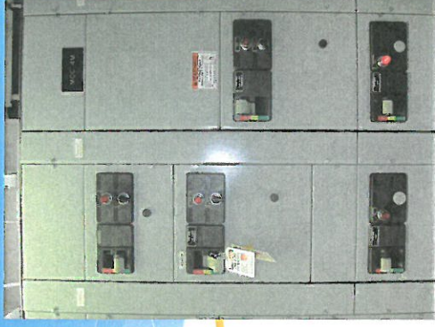
Switchgear at RP-1
