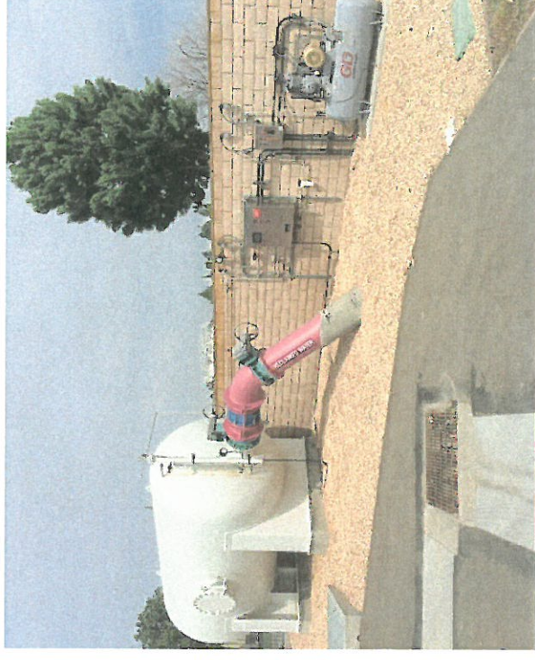
Carbon Canyon Surge Tank
