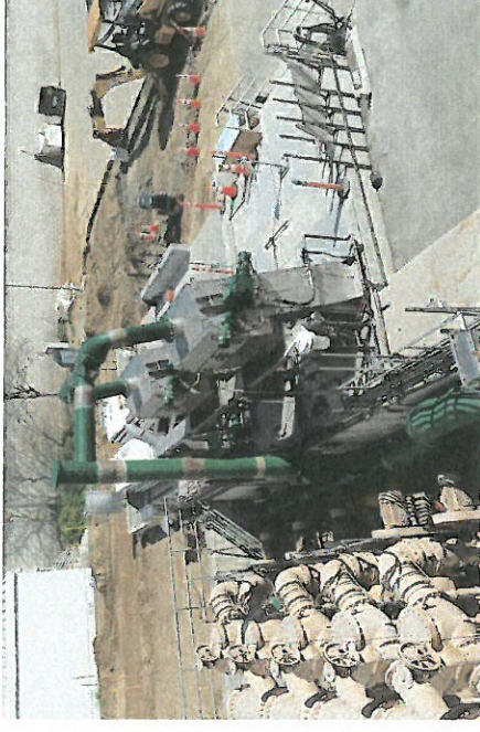
Completed Headworks Equipment
