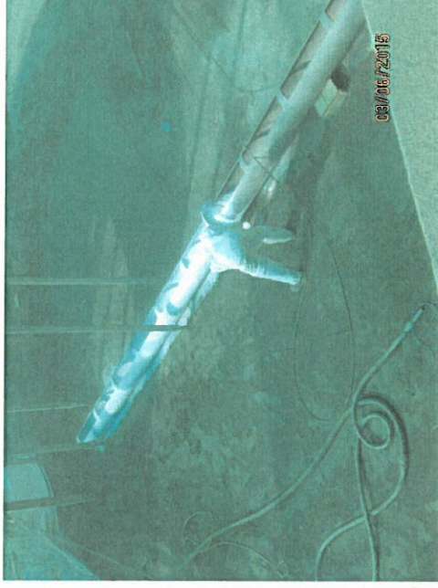
Coating of Scum Trough
