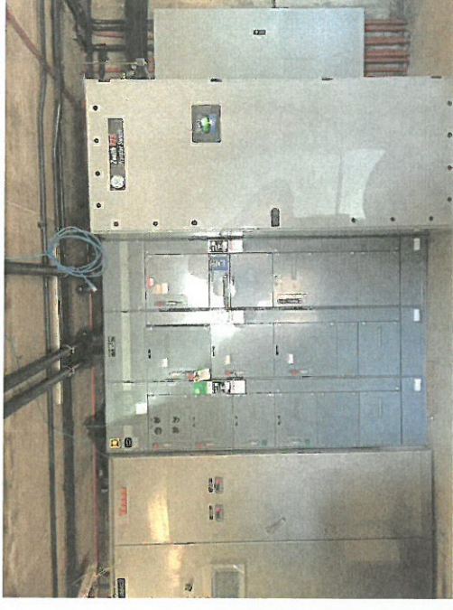
Montclair New Electrical Panel
