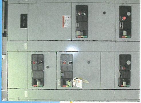
Switchgear at RP-1
