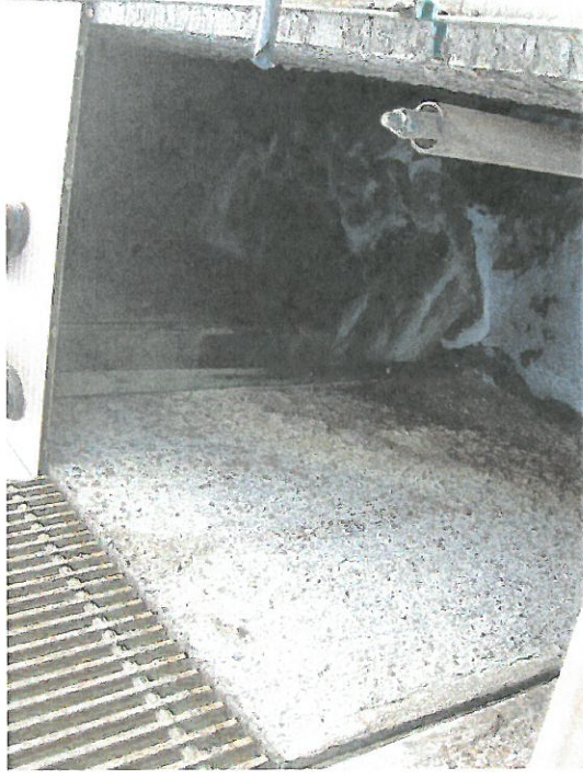
Primary Clarifier Flow
