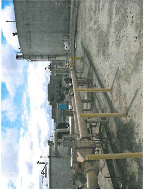
Partial DG Piping
