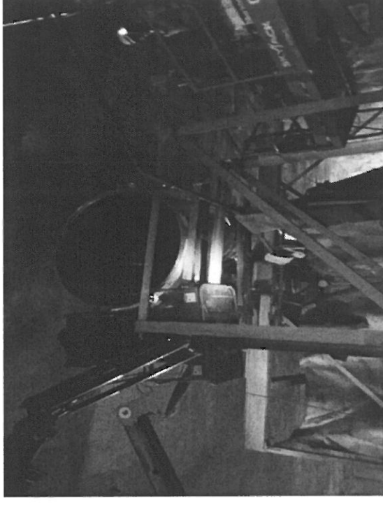
Main Dust Collecting Header
