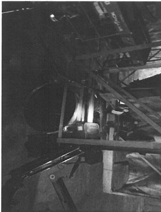
Main Dust Collecting Header
